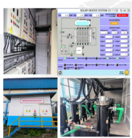
Project : Heater for Solar energy to Boiler
