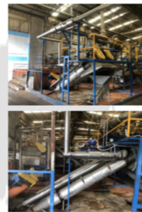
Project : Boiling process and Control Valve
